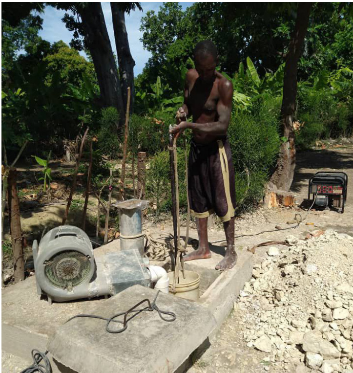
A blower delivering fresh air to a digger
